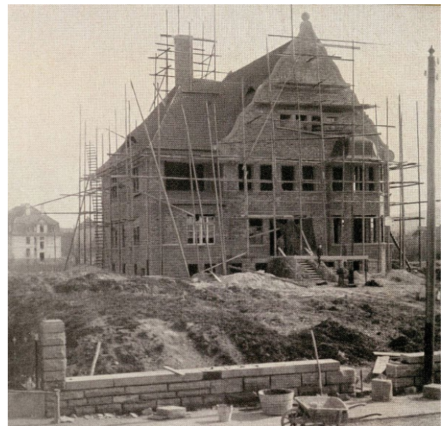
The villa, the new large residential house located diagonally across from the birdhouse on Kalandstraße, under construction.
