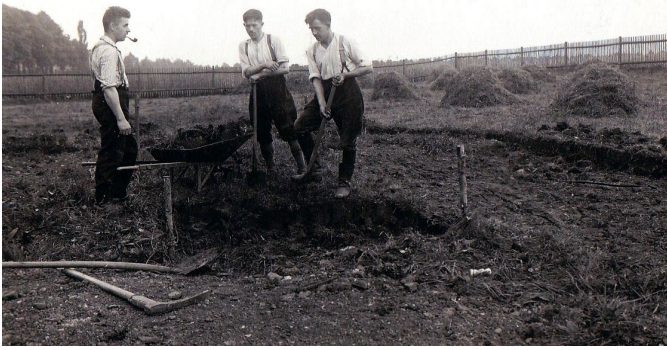
At the outset, it was difficult for anyone to imagine how attractive the pond installations would later become.
