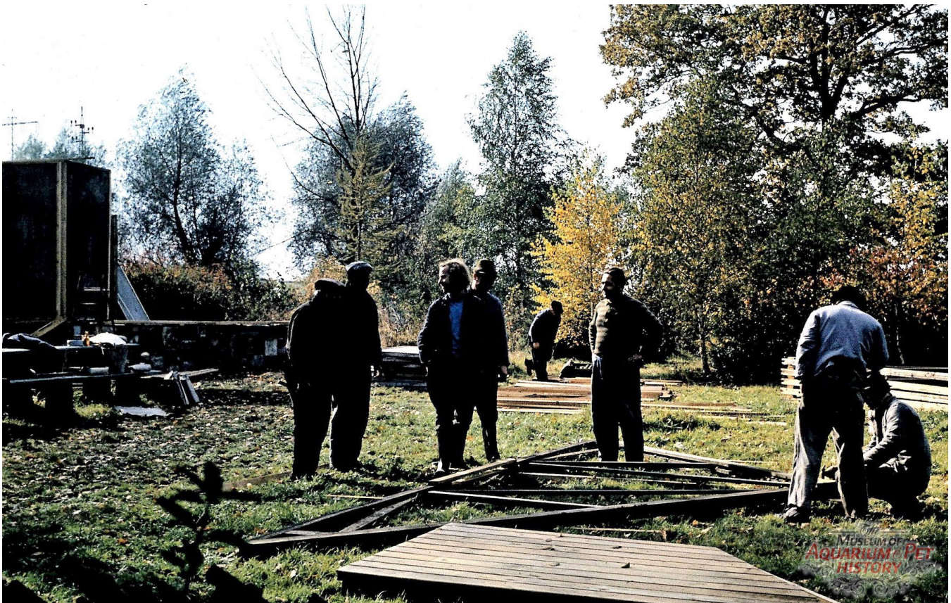
Prefabricated parts are assembled to create the barrack-like structure intended as the future clubhouse.
